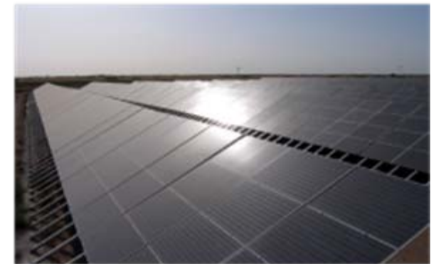
5 MW · G.E.S., Valverdon, Salamanca, Spain.
