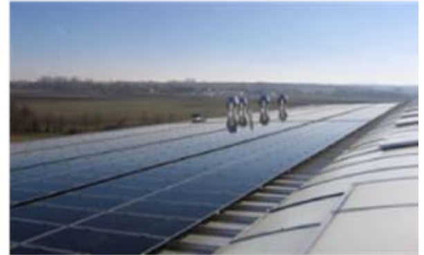
600 kW · Photovoltaic installation on the roof, Bavaria, Germany.
